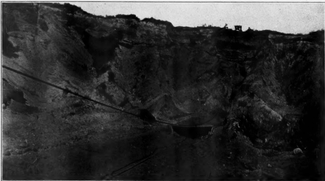
Drag Line Scraper in Operation in Sand and Gravel Pit. Cedar Grove
